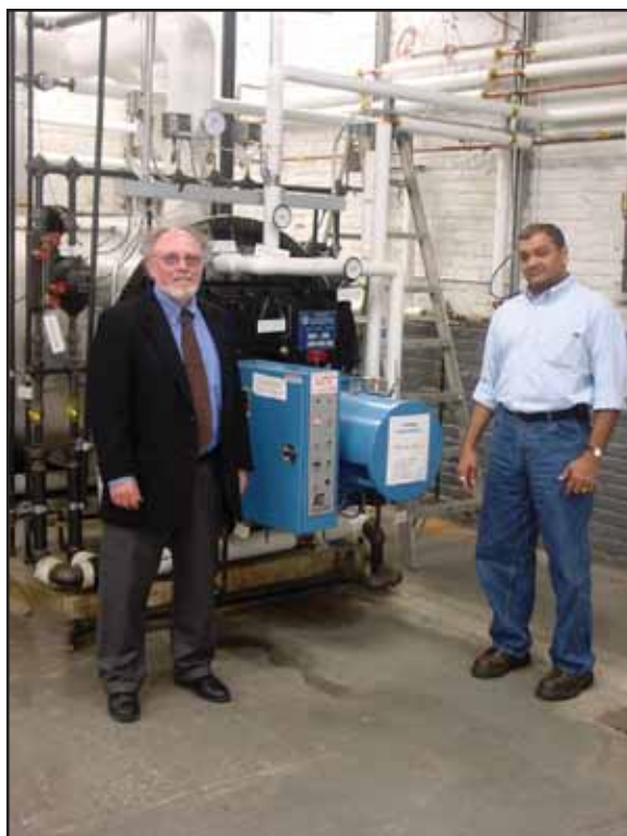
Association for Energy Affordability, Inc.'s Executive Director David Hepinstall and Chief Trainer Asit Patel in new training lab at the Energy Management Training Center
